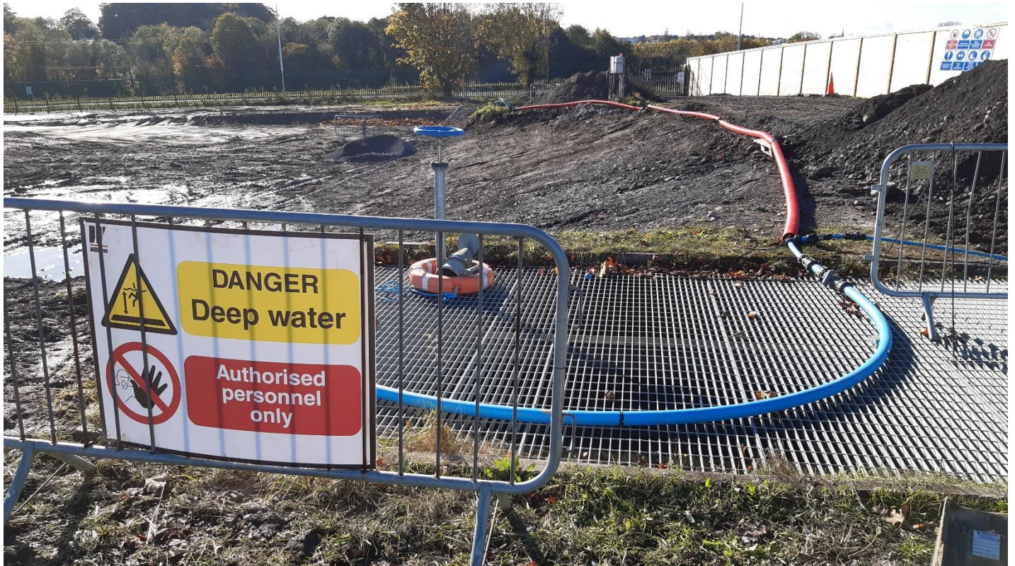
Figure 7-4 Water Sources on site
