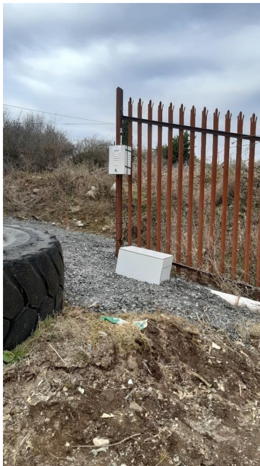
Figure 8-1 Dust Monitor - Zone 2A
